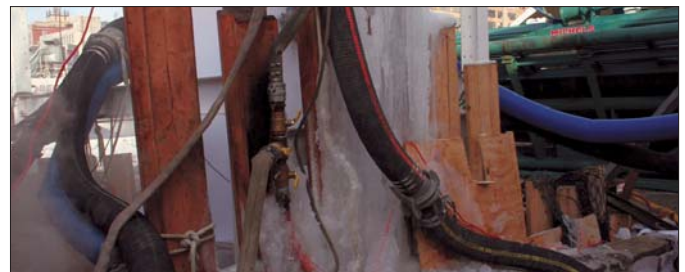
Weather was a huge factor during the project. At times, trucks and other equipment rolled to the site covered in ice.
